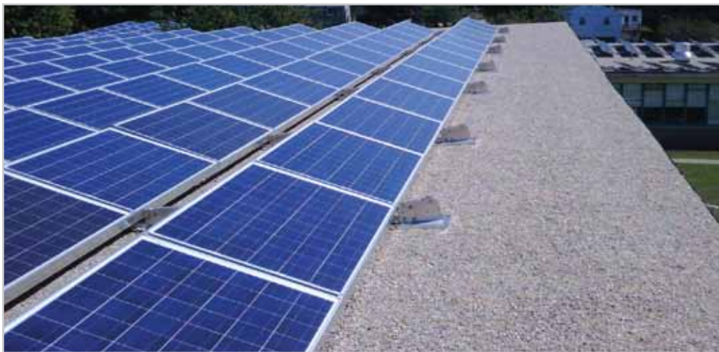
The rooftop solar photovoltaic (PV) installation at the Rellily Elementary School. The PV installations Ameresco will complete across the City will total 2.2 MW.
